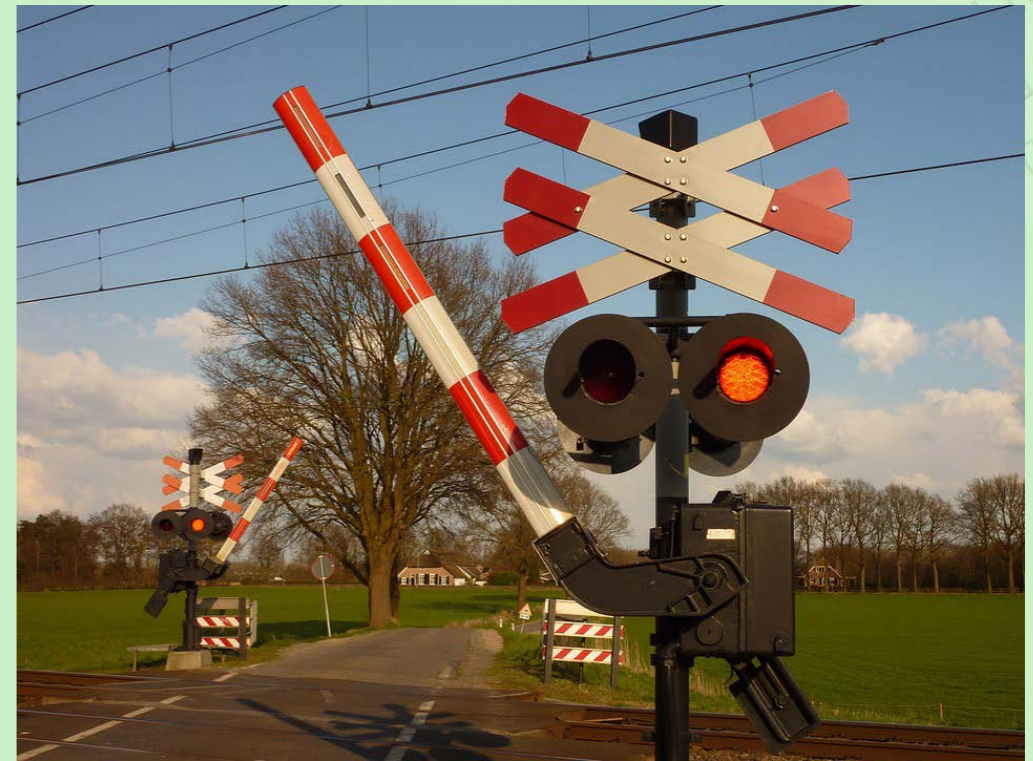
Figure 129. Railway crossing signal gates
